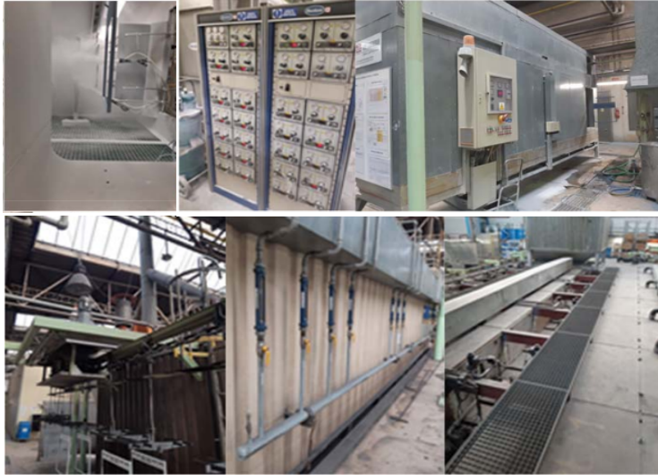
Figure 4 - Spraying cabin (top image) and furnace (bottom image).
